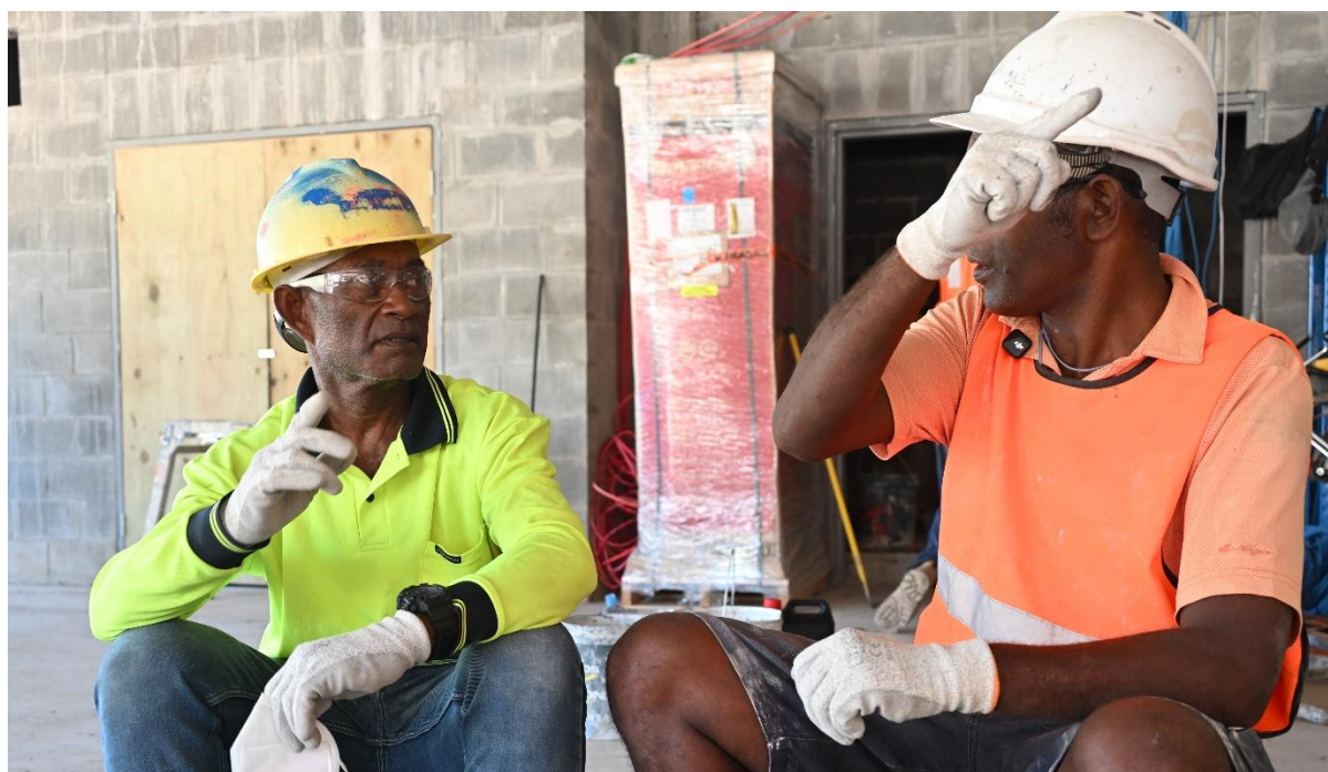
Photo 1 - Patrick Sali (Left) uses sign language to communicate with his team while completing plasterwork at the Naha Birthing and Urban Health Centre.
